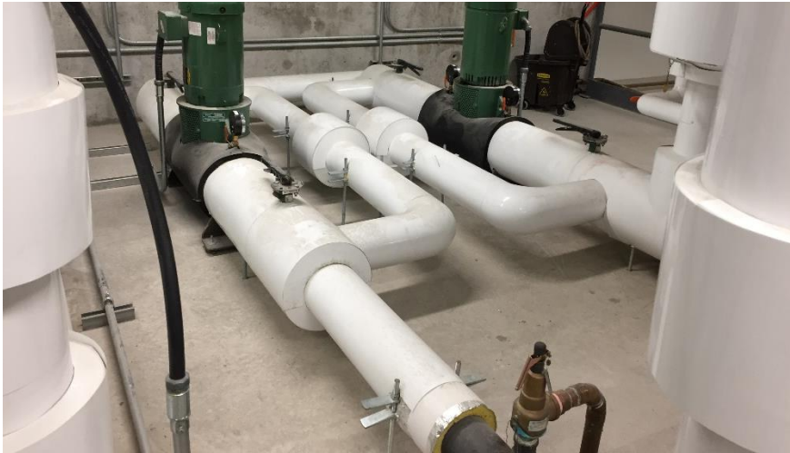
Photo 7: A typical view of fiberglass mechanical insulation was observed throughout the subject building.
