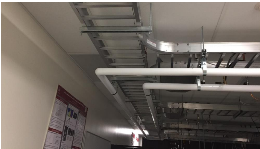
Photo 8: A typical view of fiberglass mechanical insulation was observed throughout the subject building.
