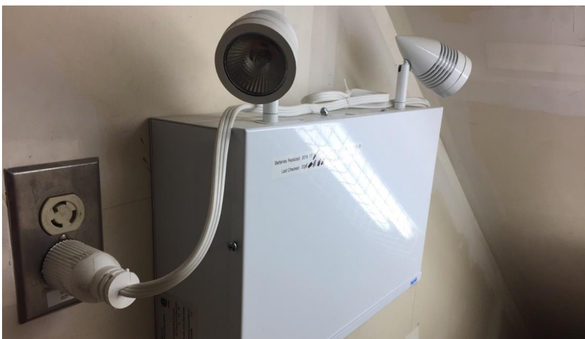
Photo 6: View of the lead-containing battery pack identified in Room 100C.
